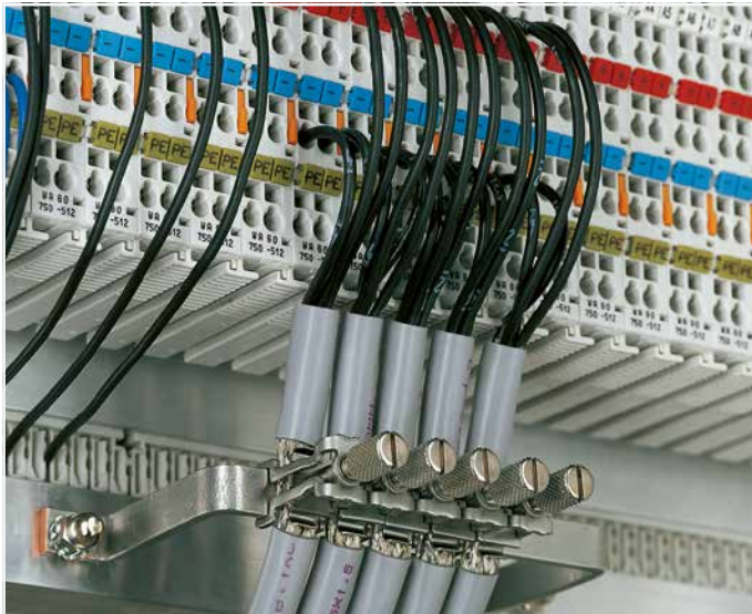
U-shaped (10 x 3) mm copper busbar
