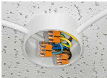
Lighting distribution in ceiling canopy
