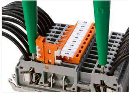
Testing with voltage tester.
