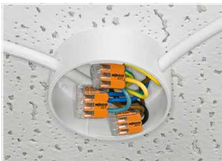
Lighting distribution in ceiling canopy
