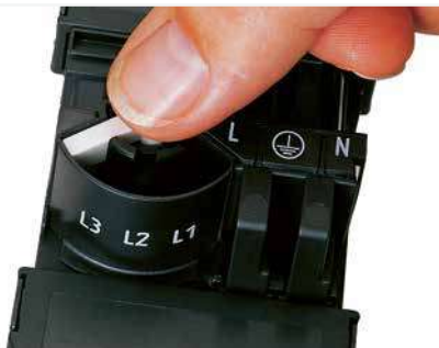
Push down jumper in its new position (picture shows L3).
